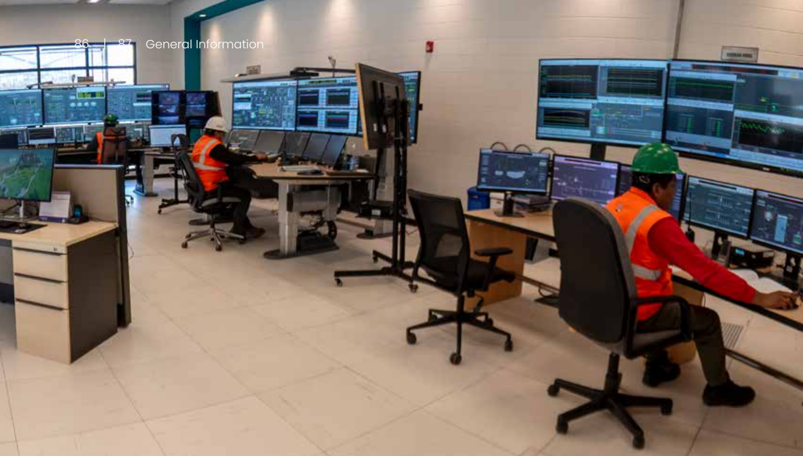
Control Room, C2 Concentrator, Toquepala, Tacna, Peru
